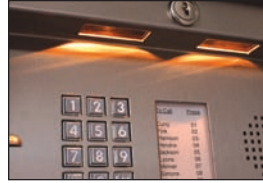
led lighting illuminates keypad and directory
